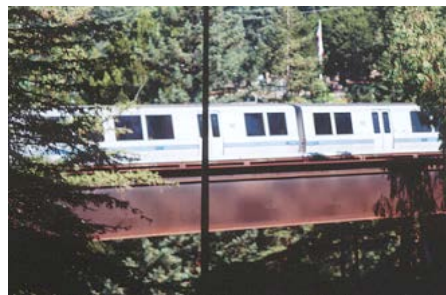
One set of BART WEATHERING STEEL TWIN STEEL BRIDGES - BERKELEY, CALIFORNIA (four total built in 1972 - 100 ft simple spans
