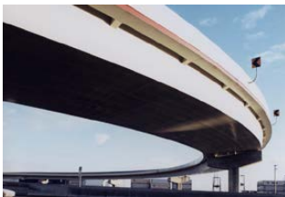
2) MARITIME OFF-RAMP I-880 OAKLAND CALIFORNIA, beside SFOBB Toll Plaza photo By Bob Collin Photographer of Caltrans
